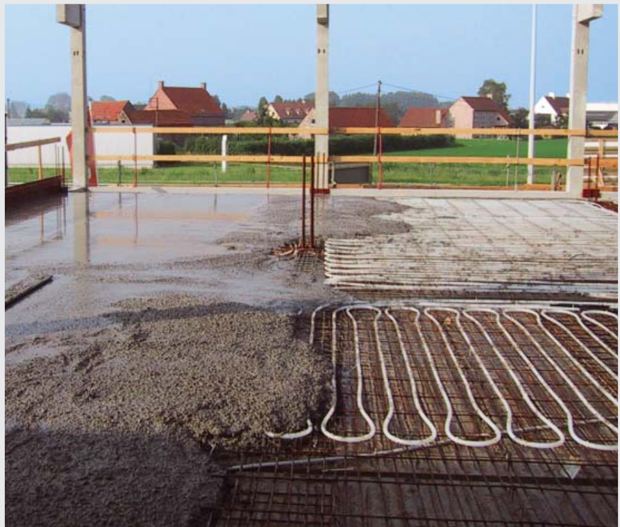
Fig. 11: Using a building component/concrete core – creating an intermediate layer with pipe system
